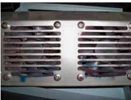
Heat is the enemy of all electronics so keep fans and cooling systems clean.
